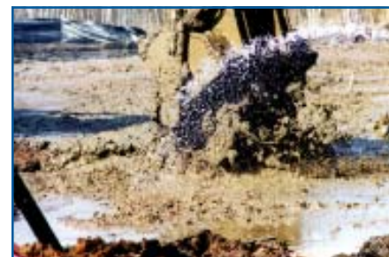
Water added as needed during mixing operations to improve homogeneity of cement-soil mixture.
